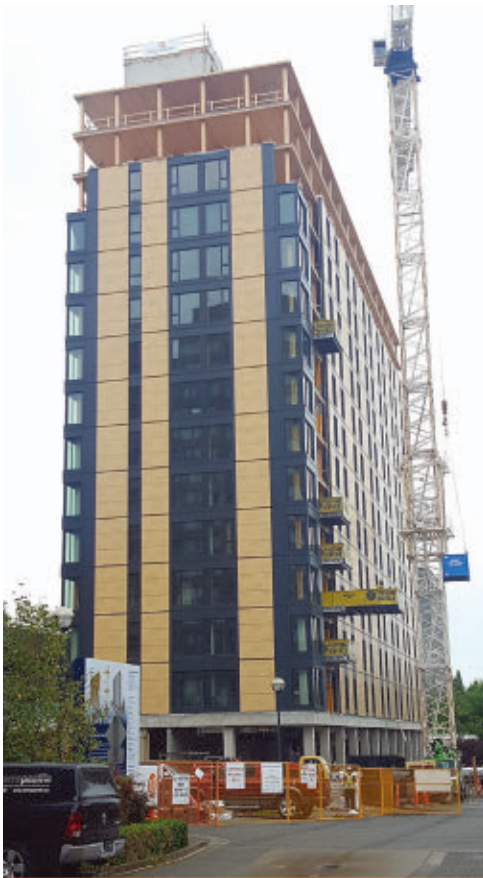
The 18-story Brock Commons at the University of British Columbia (shown here under construction in fall 2016) will be the world’s tallest building constructed with cross-laminated timber (CLT). It will house approximately 400 students when it opens in September 2017.
