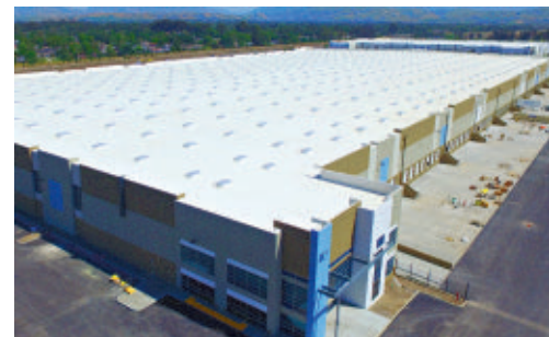
800 4x8 SKYPRO Polycarbonate Skylights and UL Listed Smoke Vents GC: Swinerton Builders City: Livermore, CA
