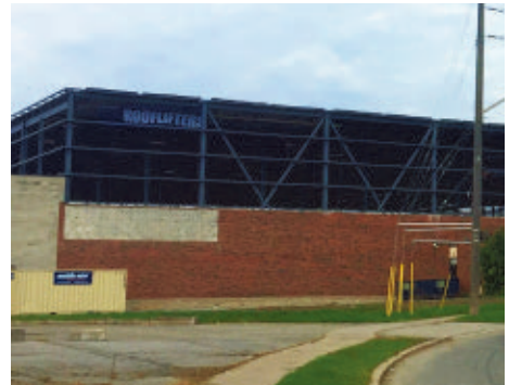
The Aurora Foods building in Toronto, Canada, just after the roof was raised from 18 feet to 40 feet. This more than doubled the cubic space of the 100,000-square-foot facility.
