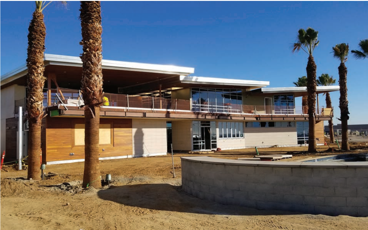
The pool building is under construction at the Costa Vista RV Park, which is part of the Chula Vista Bayfront development near San Diego.
