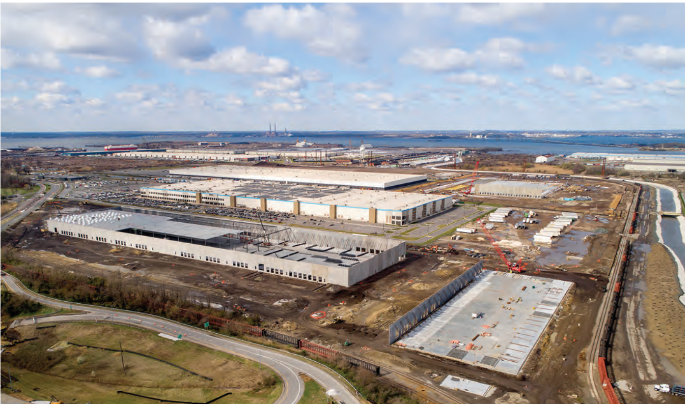
Construction continues at Baltimore’s Tradepoint Atlantic, 3,300-acre global logistics hub that eventually will be one of the largest in the country.
